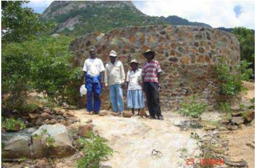
Water storage tank under construction in Nyatondo Village. Water will be piped from a reservoir uphill to be stored in the tank. Four committee members stand in front of the tank.
